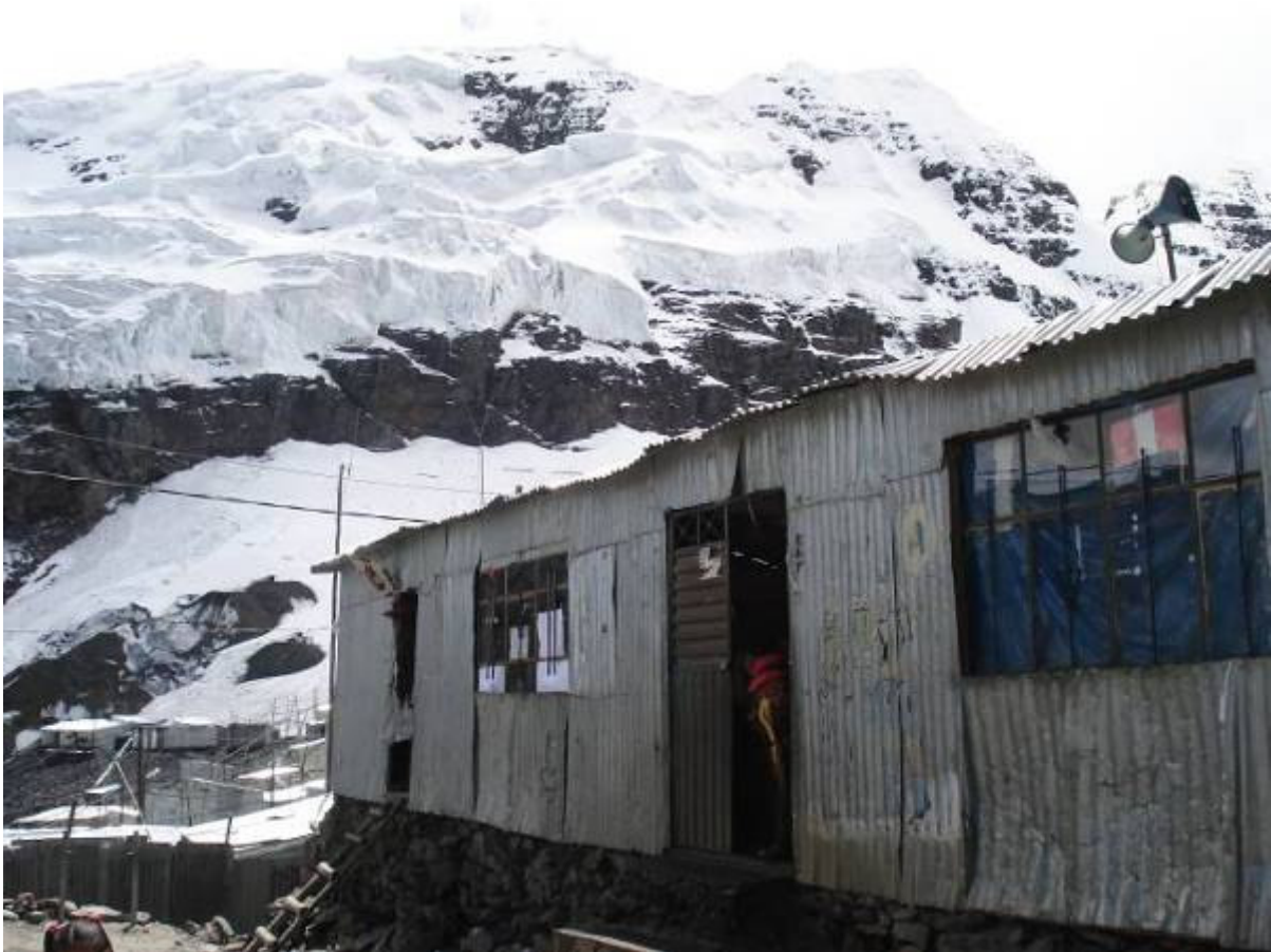
Photo 1: The poorly constructed school in La Rinconada barely shelters children from the cold
